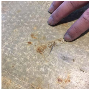
1 | A damage is discovered.
